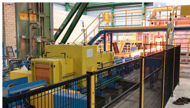
Fig. 1. Descaler equipment in charge of primary scale removal.
